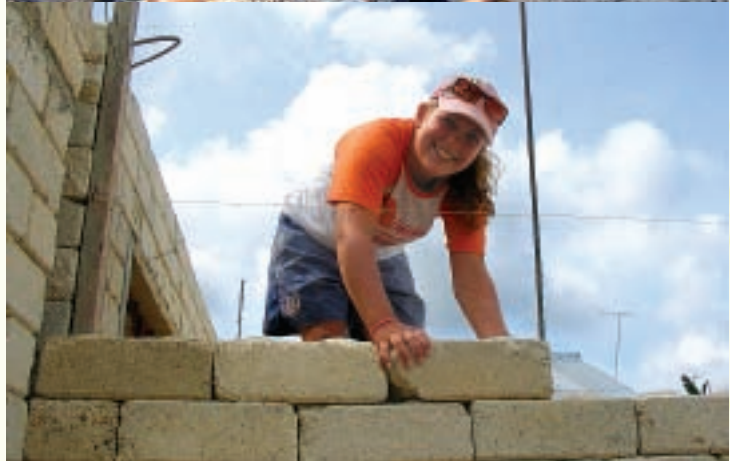
Top: New College team on site. Bottom: New resident Amy Gibbens builds a wall.
